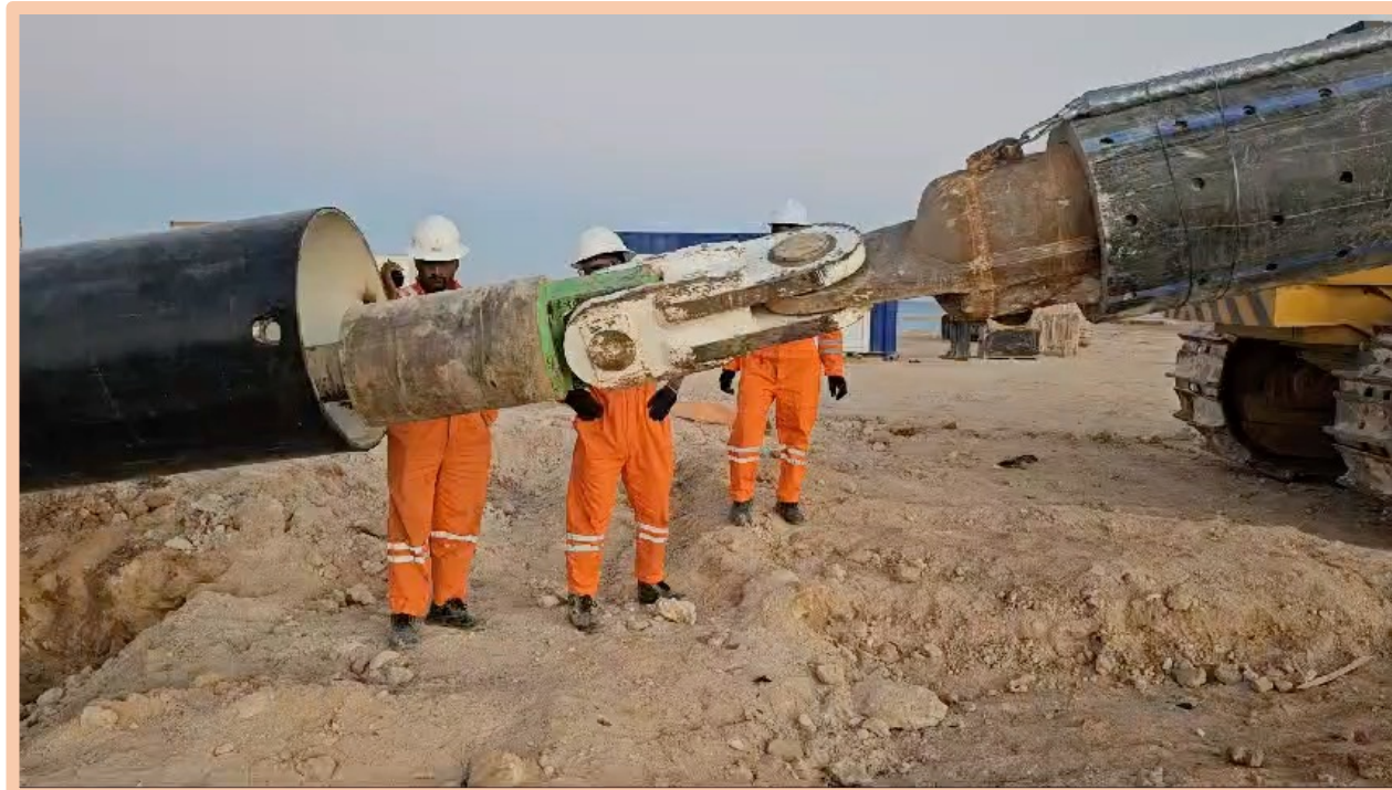
Installation of 24” HDPE pipe along with conduits inside the 32” steel casing pipe
